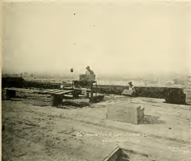
FIG. 126.—ERECTING CORKBOARD IN ASPHALT CEMENT TO ASPHALT PRIMED CONCRETE WALL SURFACES.—NOTE THE ASPHALT PAN AND OIL STOVE ARRANGEMENT FOR HOLDING ODORLESS ASPHALT AT THE CORRECT TEMPERATURE AT POINT OF ERECTION.
