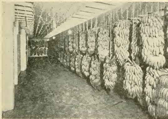
FIG. 69.—INSULATED BANANA ROOM EQUIPPED WITH OVERHEAD BUNKERS AND PATENTED CONTROL SYSTEM.
