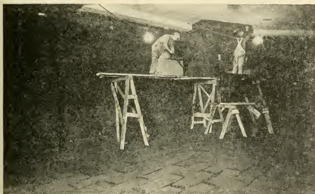
FIG. 128.—ERECTING FIRST LAYER CORKBOARD AGAINST CONCRETE WALLS, COLUMNS AND COLUMN CAPS IN ASPHALT CEMENT TO SUITABLY PRIMED SURFACES.—NOTE PRIMED BUT UNINSULATED WALL AND COLUMN SECTION AT TOP LEFT.
