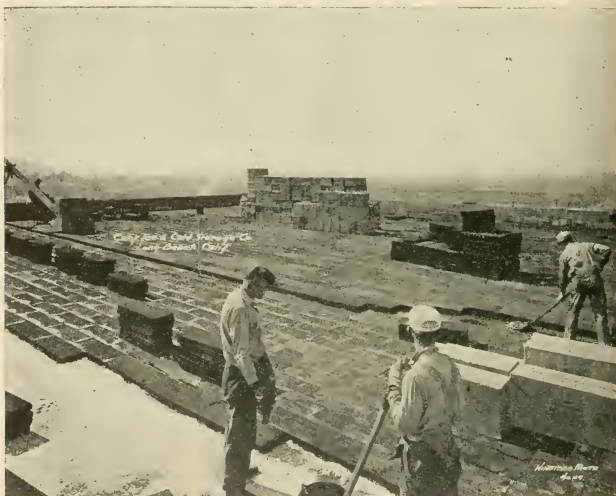
FIG. 133.—APPLYING FIRST AND SECOND LAYERS CORKBOARD SIMULTANEOUSLY OVER CONCRETE ROOF IN ASPHALT CEMENT.
