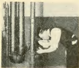
FIG. 224.—CORK PIPE COVERING ON THE LINES OF A REFRIGERATED DRINKING WATER SYSTEM.
