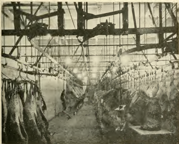
FIG. 67.—MEAT STORAGE COOLER WITH OVERHEAD TRACKING AND COIL ROOM ABOVE.
