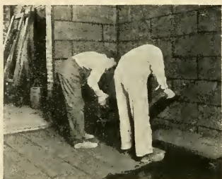
FIG. 139.—LAYING SECOND LAYER CORKBOARD ON FLOOR IN ASPHALT CEMENT—TANK BOTTOM INSULATION IS APPLIED IN SAME MANNER.
