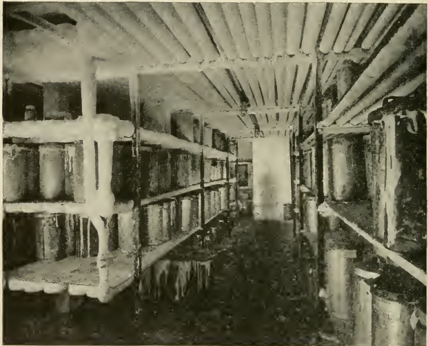
FIG. 59.—ICE CREAM HARDENING ROOM WITH PERFORATED PLATES OVER PIPE SHELVES.
