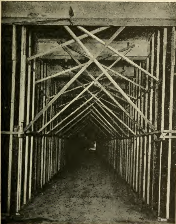
FIG. 137.—ERECTING DOUBLE LAYER CORKBOARD SELF-SUPPORTING PARTITIONS TO FORM CORRIDOR WALLS OF UNUSUAL HEIGHT.— NOTE TEMPORARY STUDS, WHICH ARE LATER REMOVED.
