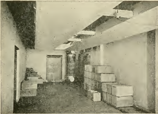
FIG 68.—INSULATED EGG STORAGE WITH OVERHEAD BUNKERS AND PATENTED VENTILATING SYSTEM.
