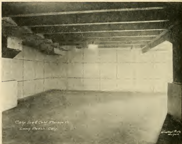
FIG. 141.—CORKBOARD INSULATED COLD STORAGE ROOM FINISHED WITH PORTLAND CEMENT PLASTER SCORED IN 4-FT. SQUARES.
